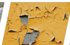
Flaking of Paint
