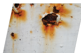
Corrosion of Steel
