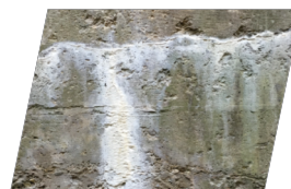
Leaching in Concrete
