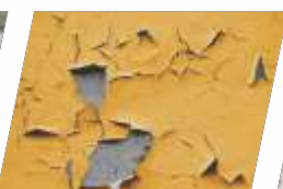
Flaking of Paint
