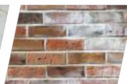
Efflorescence on Wall
