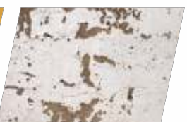
Crumbling of Plaster
