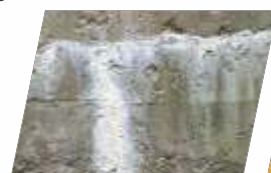
Leaching in Concrete
