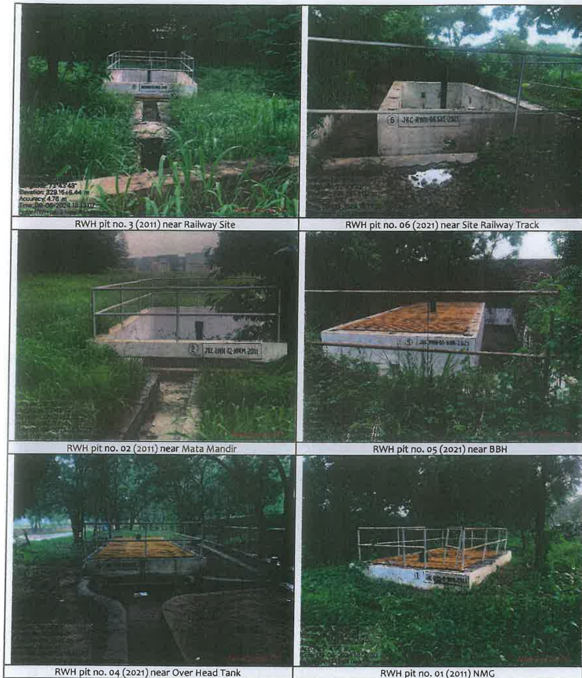
Figure 17: Photographs showing existing Rainwater Harvesting pits at the plant premises
