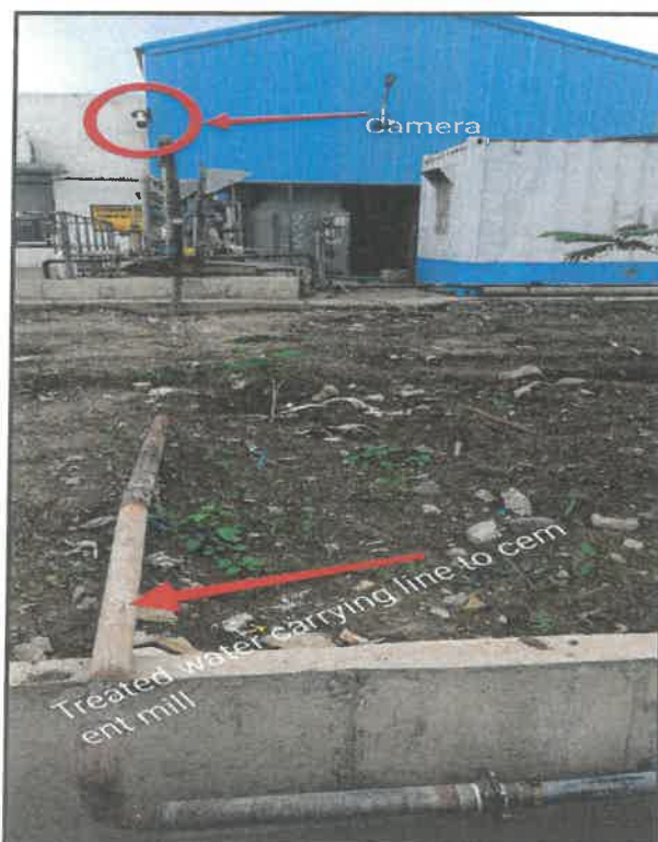
Picture 7- Camera installed at WHRS Treated water discharging point
