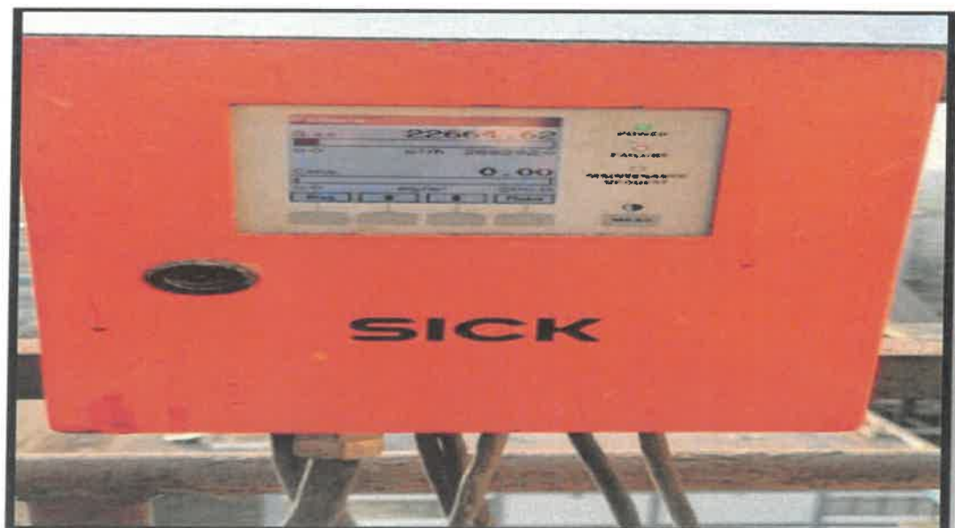
Picture 6- Continuous Emission Monitoring Systems (CEMS) installed
