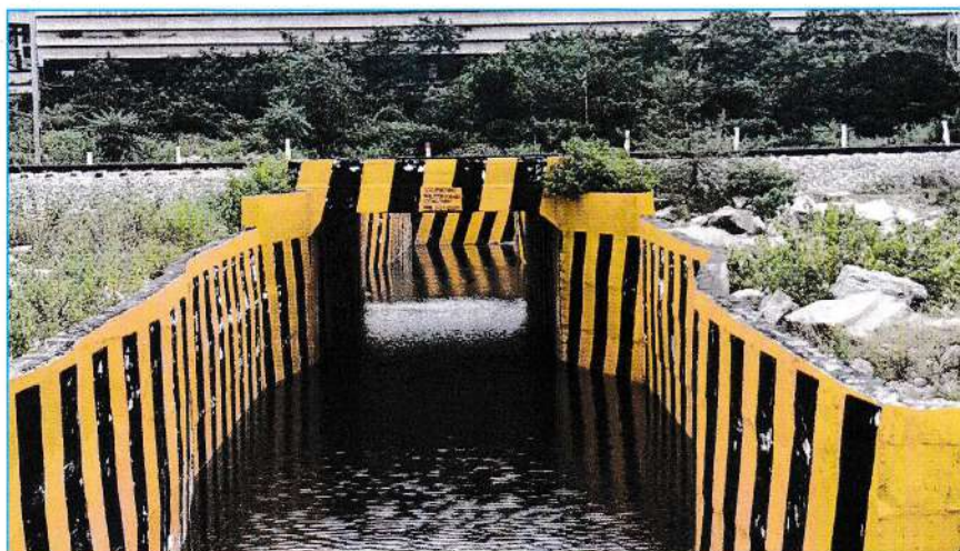
Plate 5.6. View of the underpass for road below the new & old railway lines
