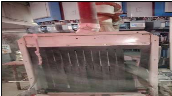
Cement Bag cleaning system
