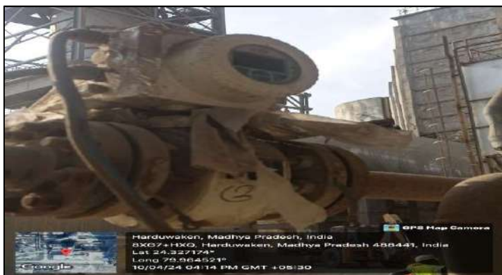
Cooler spray meter
