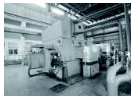
► Inside view of Mangrol Captive Power Plant
